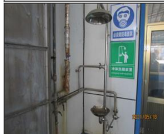
Photo first aid facilities Eye wash equipment.JPG
